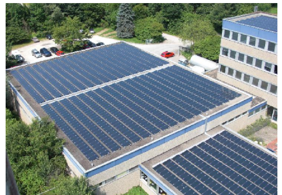
Largest FORMSOL system in Europe, Neckarhausen, GE
