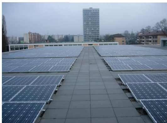
Photovoltaic system on school in Hirzenbach in Zurich
